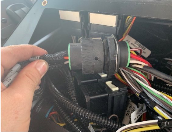
Figure 10: BB1 connected to MP92-1021
