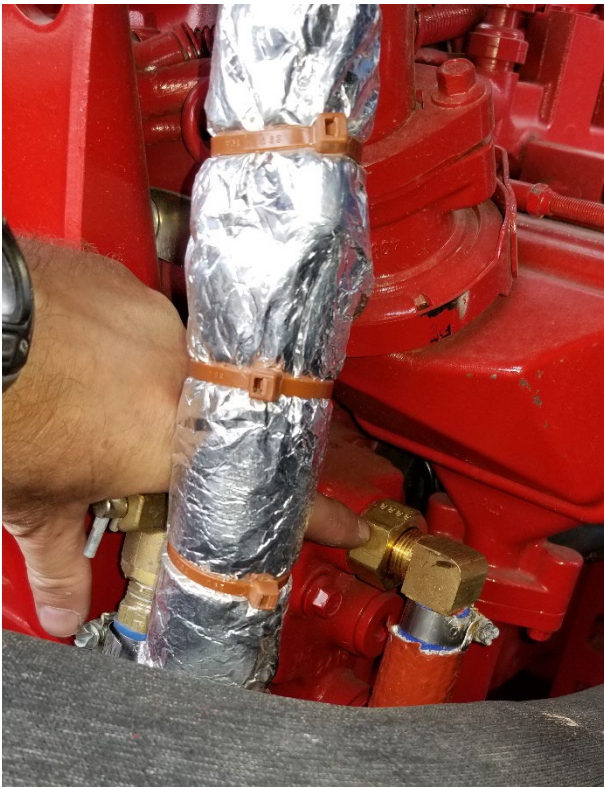
Figure 13: Coolant Supply Line on Engine Block
