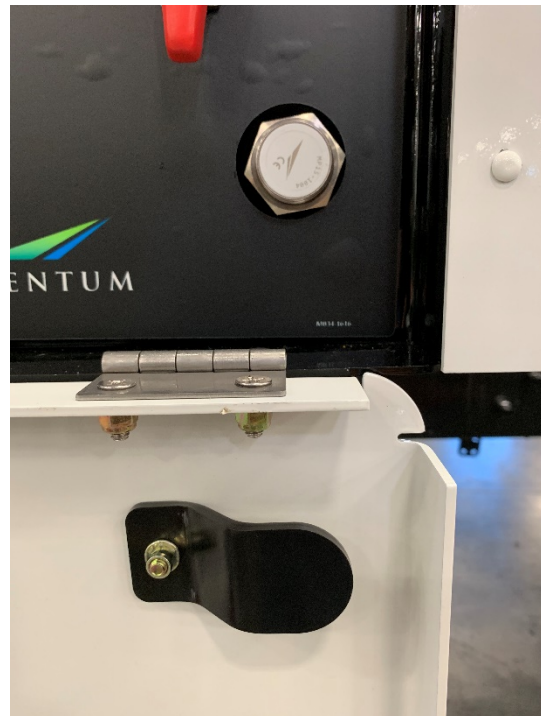
Figure 39: Start Interrupter Switch
