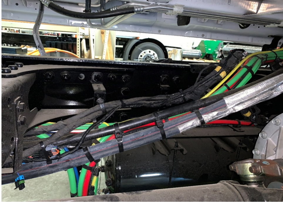
Figure 27: Wiring Harness Routing-Under Cab
