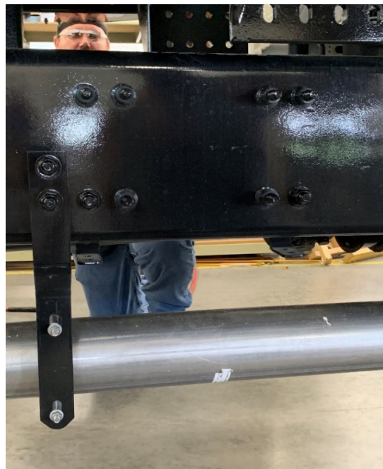
Figure 4: Huck bolts on Frame
