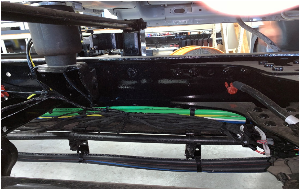
Figure 21: Wiring Harness Routing-Behind Cab
