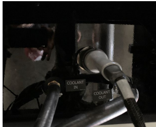
Figure 16: BOC Electrical and Coolant
