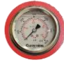
RED labeled gauge is PRD gauge indicates the cylinder pressure regardless of the valve position.
